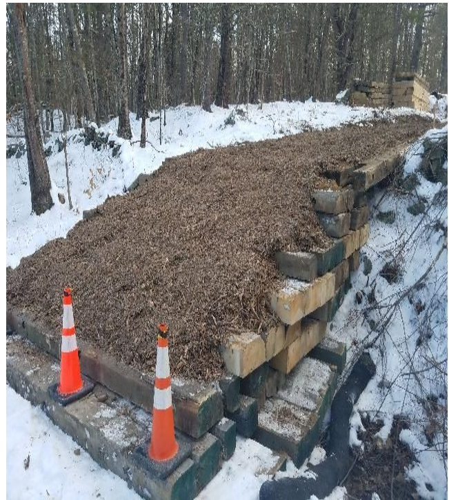
Fig 4: Access road off of Timber Brook Lane, over rock wall WP-22. Viewing northeast. (01-24-20).
