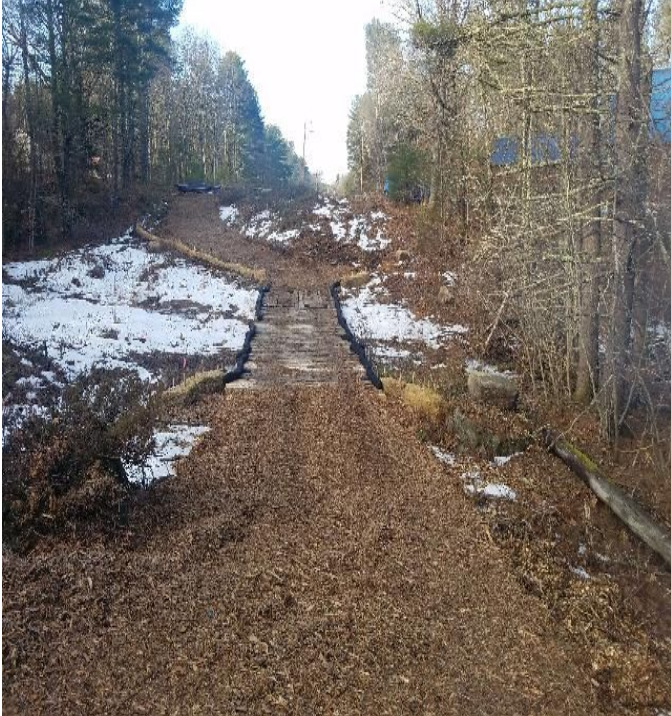
Fig 7: Access road through wetland DW9, between Strs. 65 and 66. Viewing west. Note stump grindings stabilizing slopes. (01-27-20).
