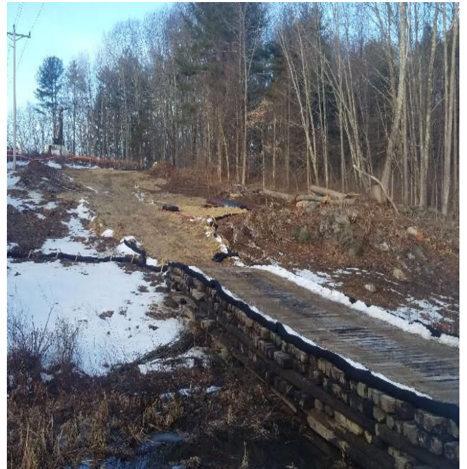
Fig 8: Access road to Str. 58 of off route 108. Bridge through wetland DW29. Viewing west. (01-27-20).
